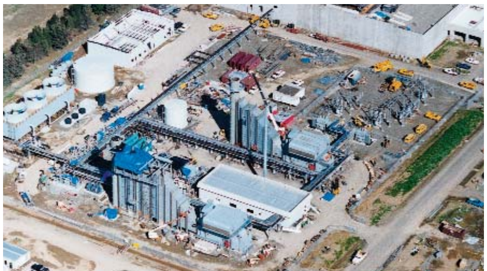
The 365-megawatt Selkirk Cogeneration Plant relies on Thermoflow software to monitor plant performance.
